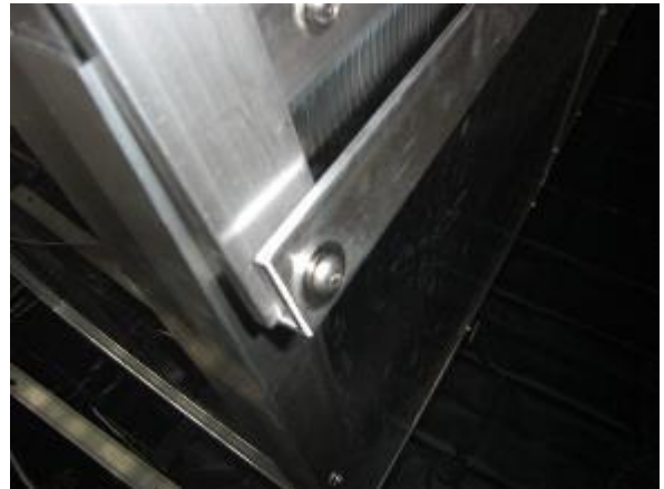
Picture 22: Fix flat aluminium bars 50x2 and 10x5mm separated in picture 19 at the side part using screws and washers. Bend plates according to the roof arching and clamp flat aluminium bar 10x5mm under them. Start parallel and uniform fixing from the bottom up together with the installation of flat aluminium bar 50x2mm at middle supports (see picture 23). Attention: only fix screws slightly
