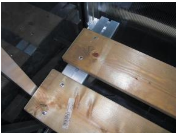
Picture 31: Adjust bench boards and distribute nuts below the bore holes of boards. Tighten with slotted screws DIN 964 M6x35.
